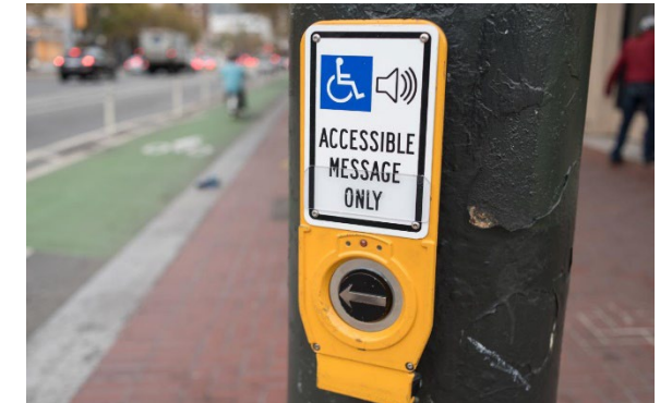
Accessible Pedestrian Signals (APS)
